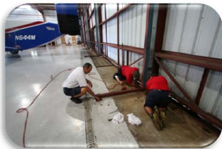
Ken Bouck, Mark Prince and Jorge Santiago secure hangar doors in preparation for hurricane Erika
